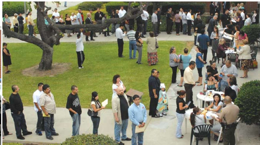
Damaged courtroom, above left, awaits repair as West Covina Courthouse personnel move service outdoors after a major water pipe burst. Clean up crews were required to remove the water and repair damage. Customers waited patiently.
